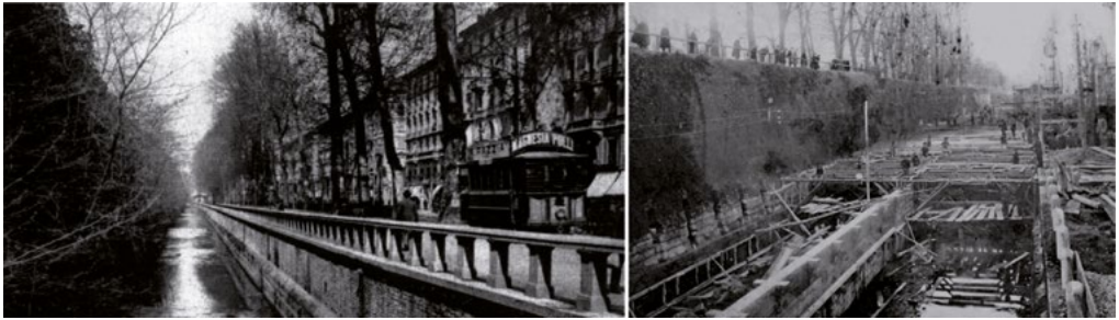
2: The section of the Redefossi canal just before it was concreted over [G. Modiano, 1899-1903] and during the covering works (1906) [Milan, Raccolta delle Stampe "Achille Bertarelli"].
